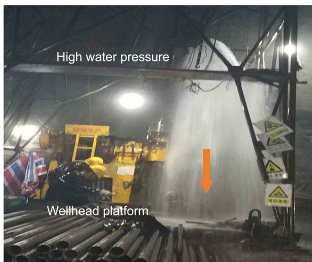
Fig. 4 High pressure water inrush during drilling
